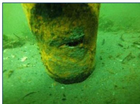
Hole in existing helical anchor is unsuitable for use.
