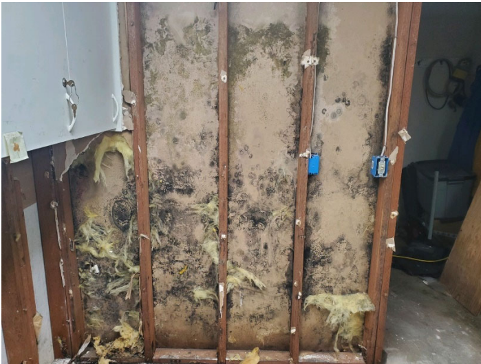
Rotted Wall with Mold
