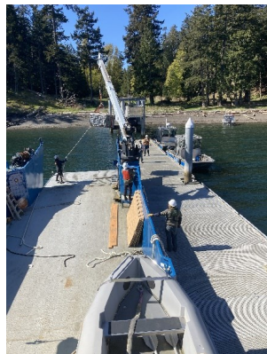
Towing docks (San Juan Islands), Backhauling equipment (Deception Pass), Spring dock installation (Jones Island)
