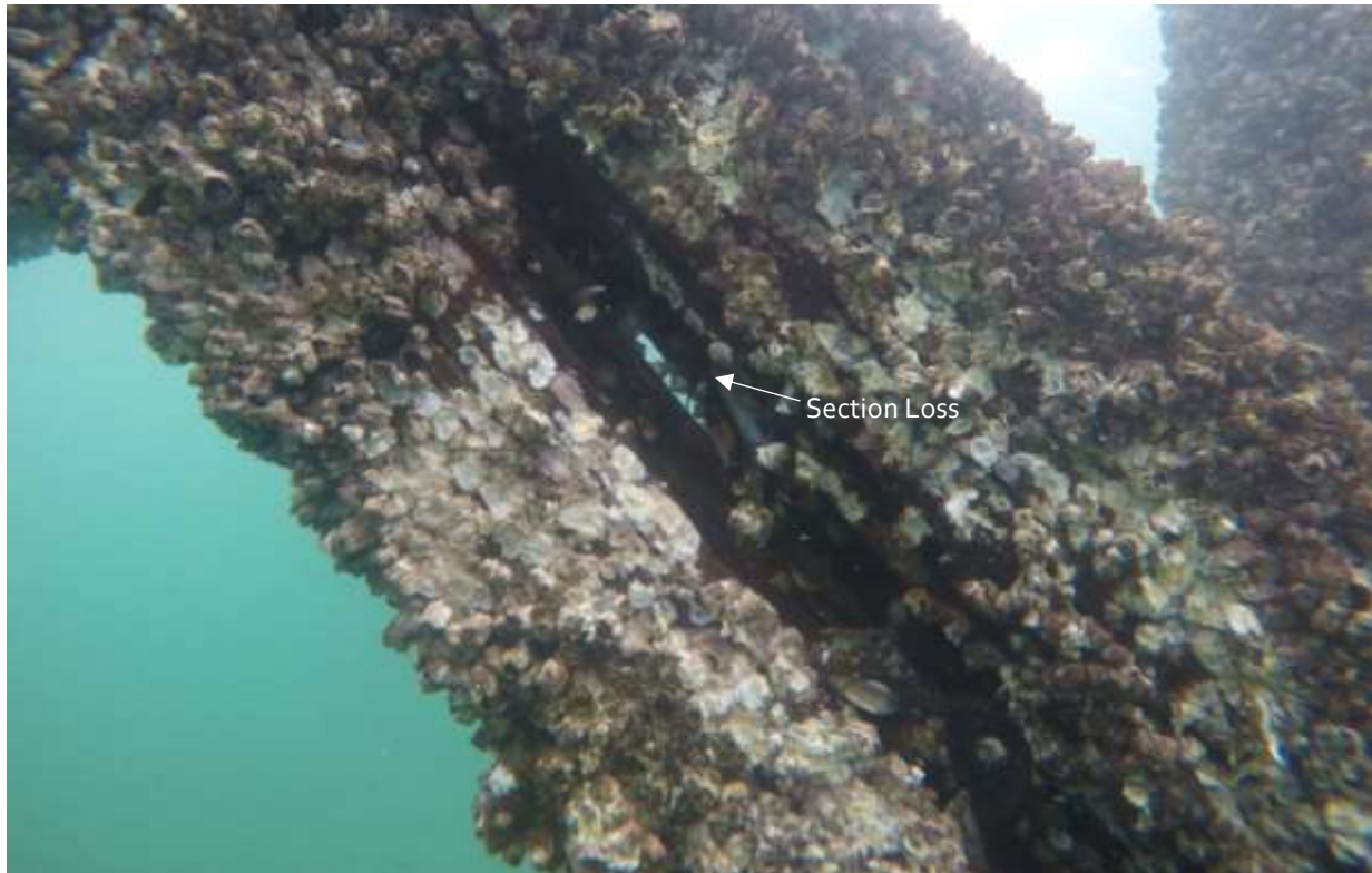
Figure 6. Cross Brace with Section Loss
